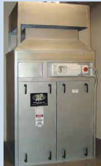
Air Tower Unit Quietly supply's air to the underfloor plenum
