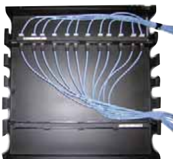
Modular Cabling (passive)
