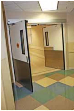
GT 500 automatic swing door operators are used throughout the facility to aide or control traffic flow and to provide security. Doors in secure areas use card readers for activation, and magnetic locks or electrified panic hardware for security. Doors in non-secure areas typically use push plate wall switches for activation.
