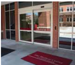
The GT 1175 single sliding entrance door at this location is fully automatic (overhead sensor activated) during the day. In the evening, a computer switches this entrance to a secure employee entrance. After hours, this automatic sliding door requires card access for entry.
