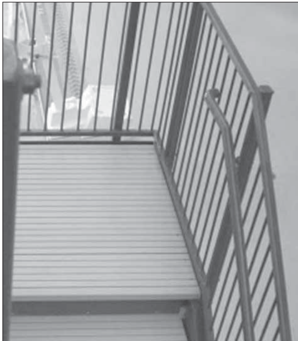
Durable, corrosion resistant Fiberglass Grating was used in construction of stairs and walkway for this outdoor environment.
