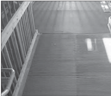
Pultruded Fiberglass Grating provides a safe walkway.
