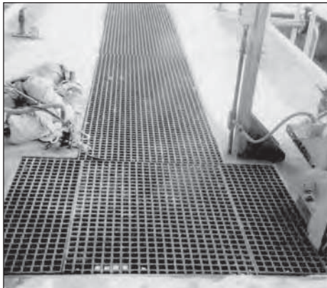
Square Molded Fiberglass used for this trench covering allows drainage.
