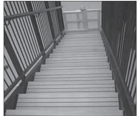
Pultruded Fiberglass Wide T-Bar Grating was used on this stairway and platform assembly.
