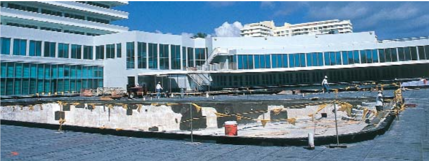
With the pool deck nearly ready for bricklayers, ProTek crewmembers work to ready the area for a leak test — in this case, complete immersion in four inches of water for 48 hours. The rubberized asphalt decking system passed with flying colors.
